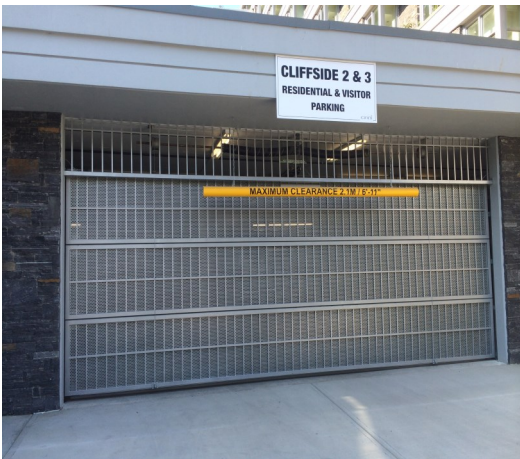
Perforated Steel Covered Main
